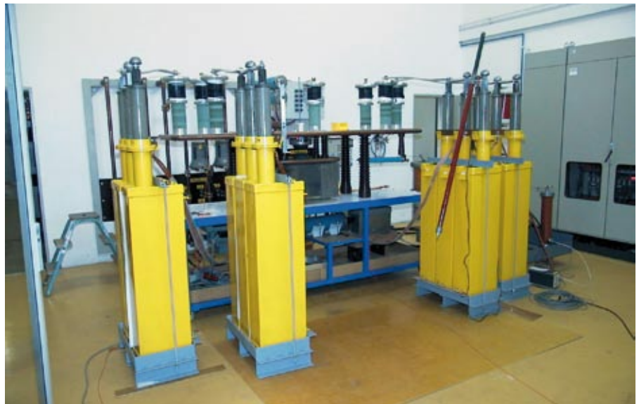
Stoßstromgenerator, Prüfstand 1/Surge generator of test room 1
